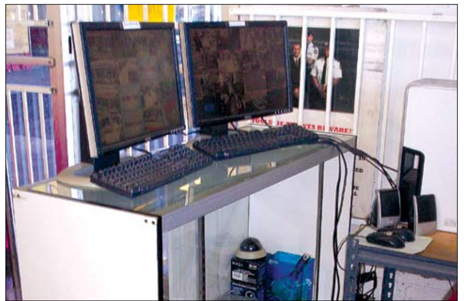
BSW uses the Geovision closed-circuit TV system. Its “payoff was priceless,” says Hoss.
